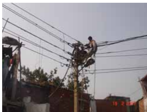
Acquiring illegal connections through hooking
